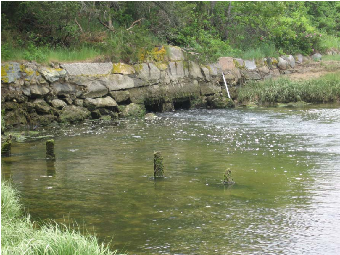
Figure 1. Pleasant Bay entrance of the existing Muddy Creek culvert. The culvert has two 3-foot-wide channels that span the 100-foot distance under the Route 28 roadway.
